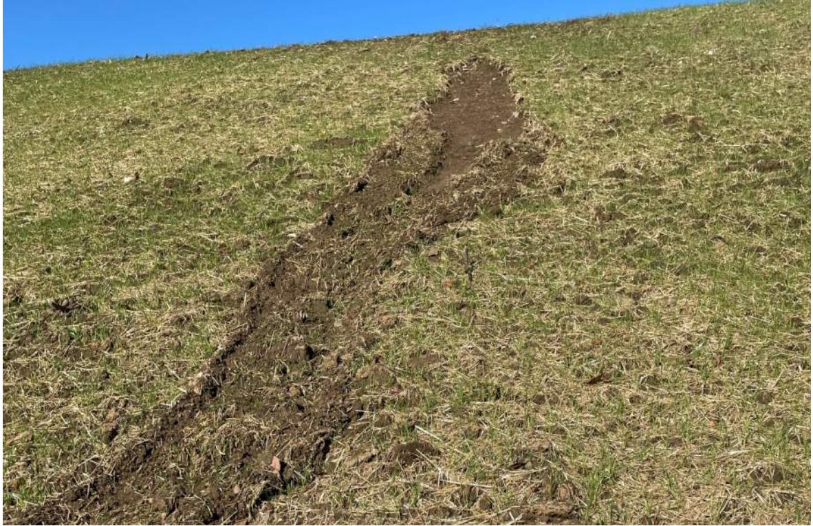
Photograph 12 – Regraded downstream side of dam below access road. Minor surface sloughing.
