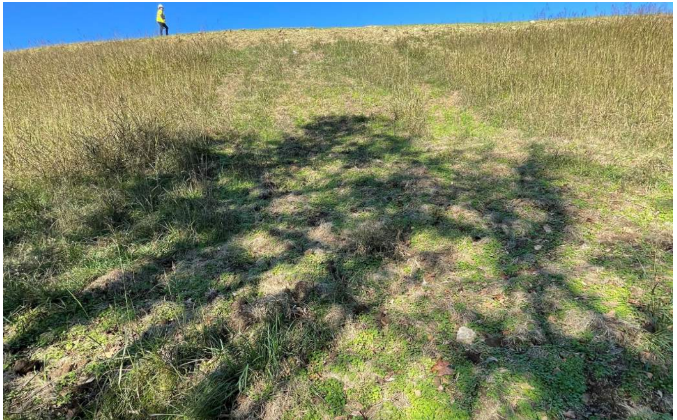
Photograph 13 – Downstream side of dam east of access road. Several areas of sparse vegetation where the bulldozer traversed the slope.
