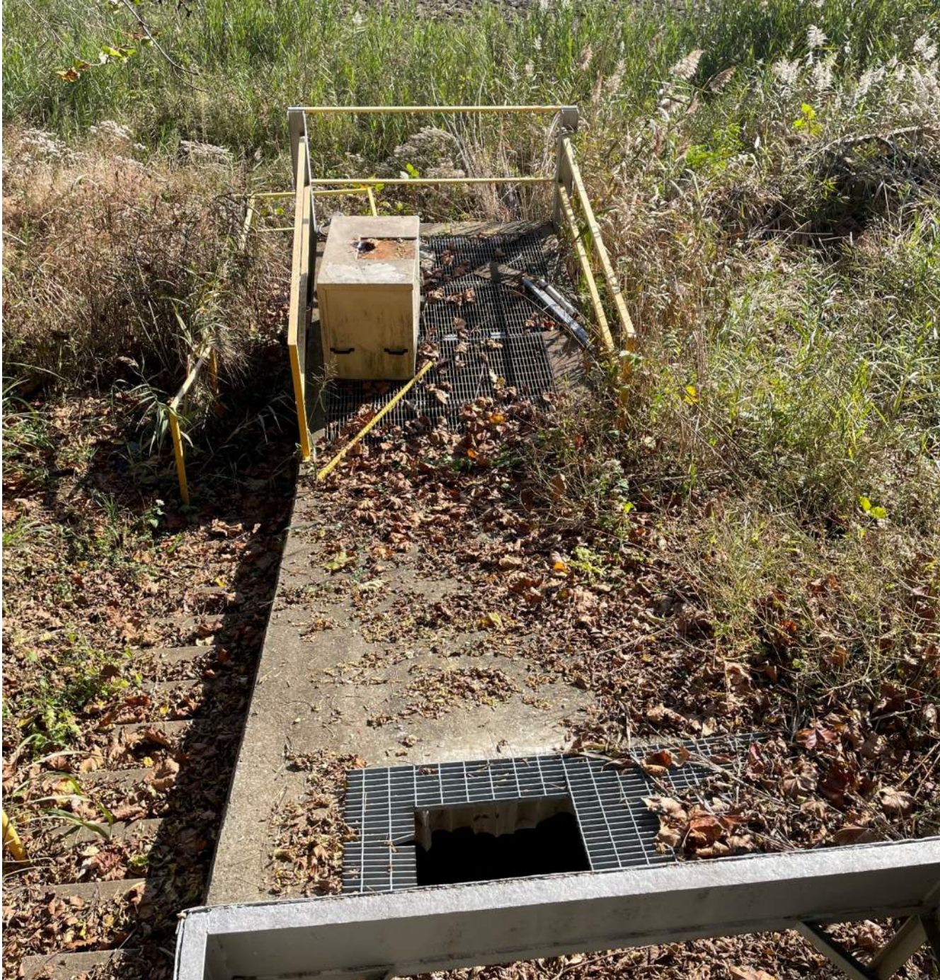
Photograph 7 – Previous inlets for Outfall 001. Access to current inlet via stairway on the left.
