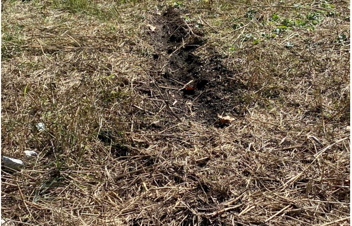
Photograph 11 – Southern dike embankment downstream side, showing erosion in damaged vegetation.
