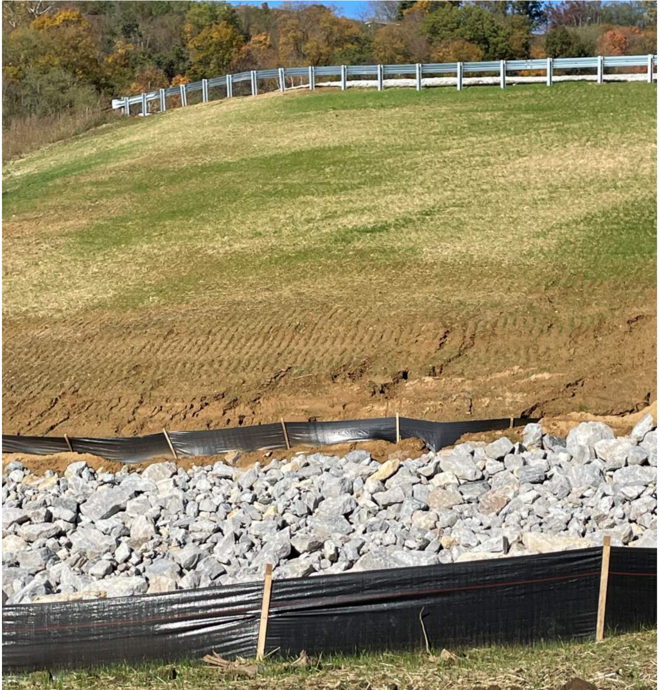
Photograph 10 – Western part of regraded downstream side of dam. Note the erosion rills forming above the channel.
