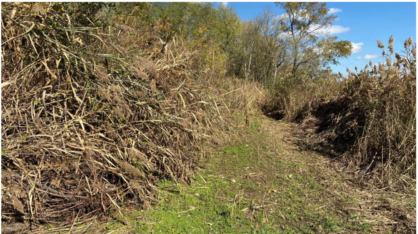
Photograph 6 – Southern dike embankment downstream side, overgrown section with trail cut in, looking east.
