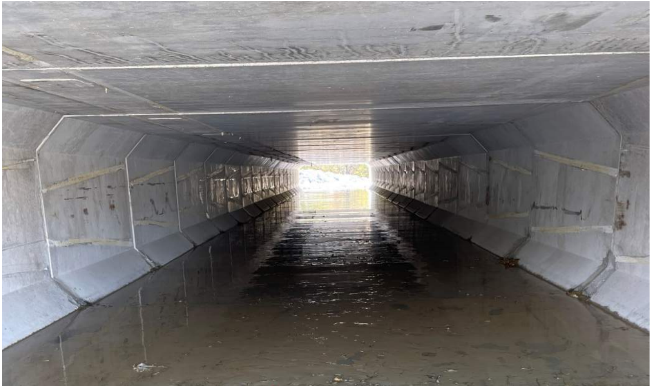
Photograph 18 – Upstream side of dam at new 12x4 culvert, looking south west through the culvert.
