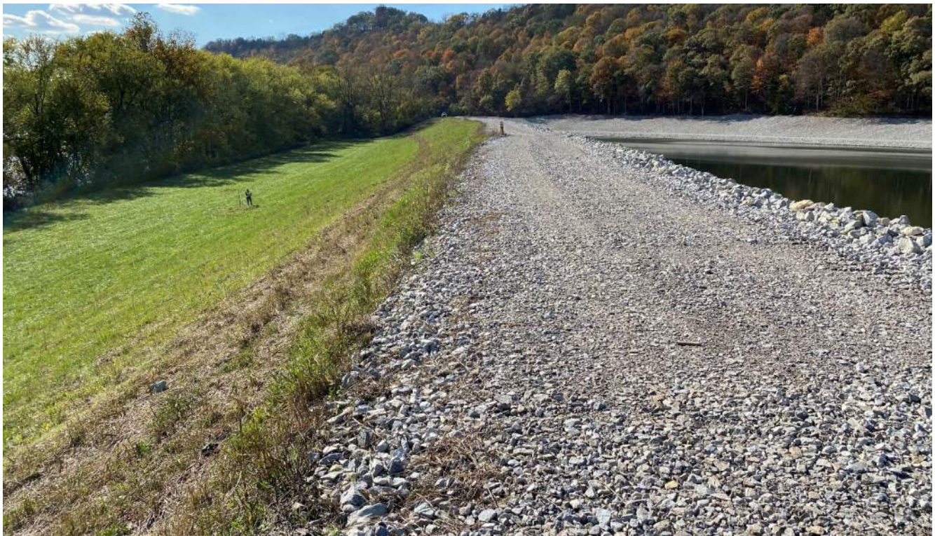
Photograph 4 – South dike embankment crest, looking west. Note the brown damaged vegetation parallel to the top of the slope.
