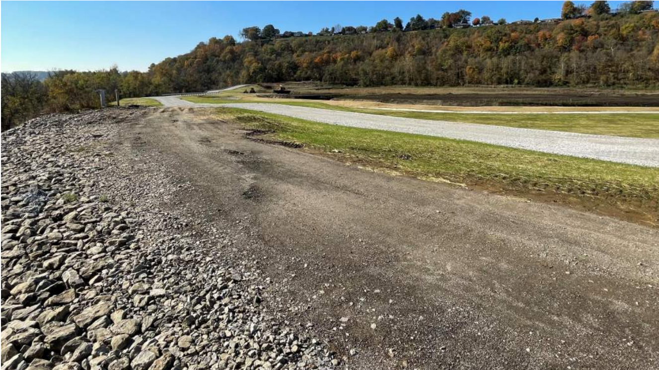
Photograph 16 – Crest of dam at the east end, looking west at the new access road and the top of the dam.
