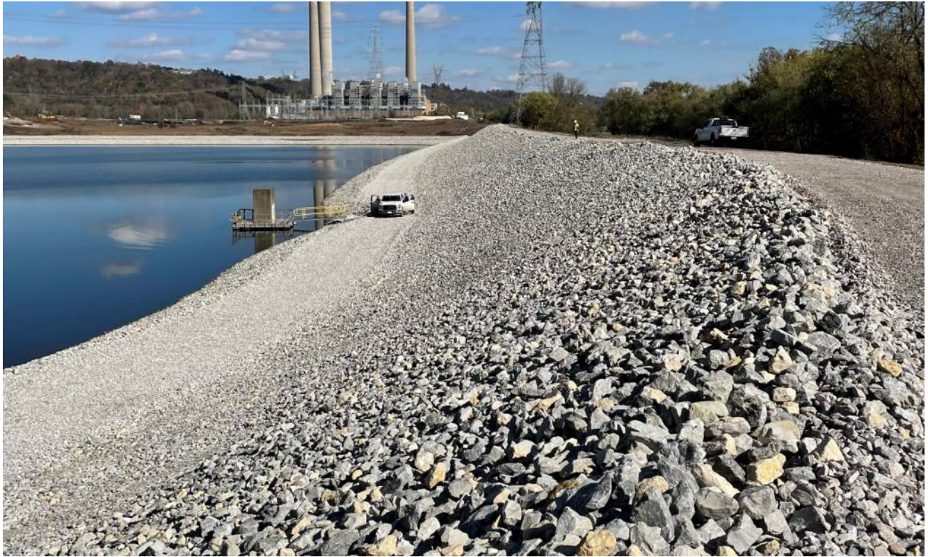
Photograph 3 – South dike embankment, upstream side looking east. Crew repairing railing around outfall structure.
