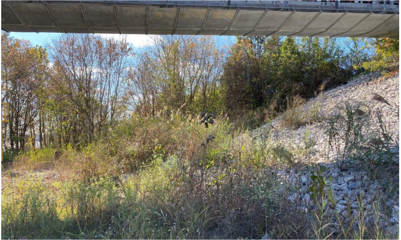
Photograph 7 – Southern dike embankment downstream side, overgrown section looking west beneath the gypsum conveyor.
