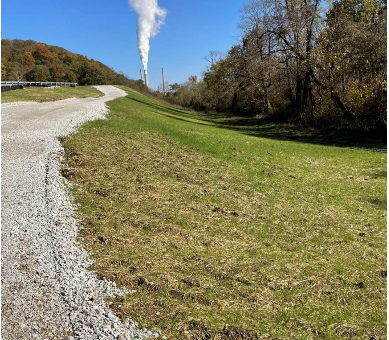
Photograph 11 – Downstream side of dam below the access road to the toe, looking east.
