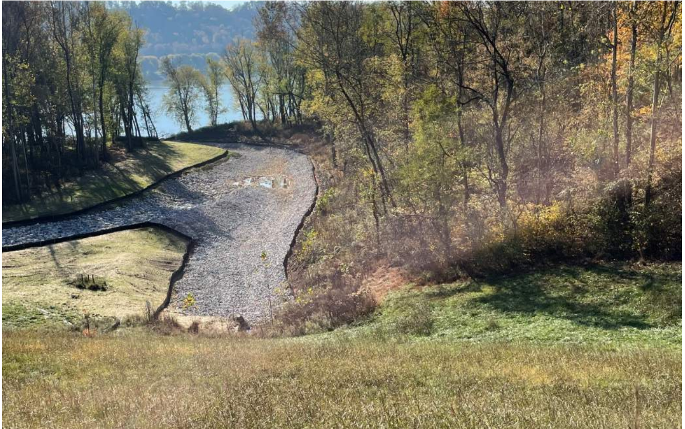
Photograph 3 – Downstream side of dam, newly constructed outfall channel to the Ohio River.
