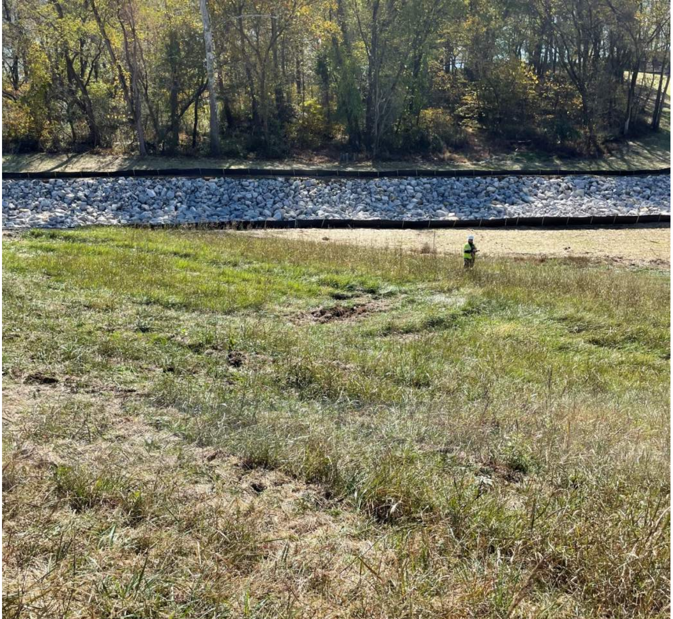
Photograph 9 – Western downstream side where the channel extends along the face and toe of the embankment. Note disturbed spots in grass from equipment.
