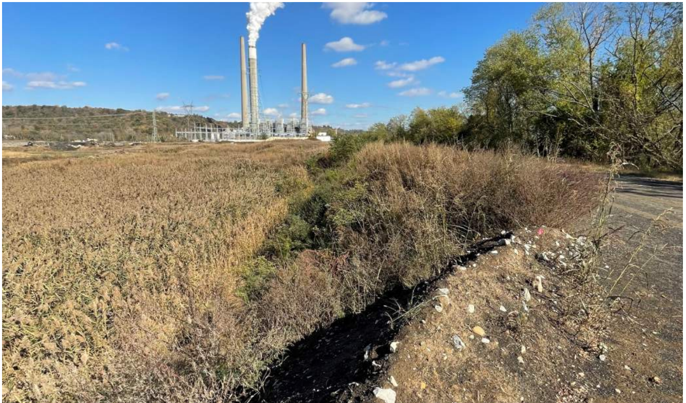
Photograph 8 – Southern dike embankment upstream side, overgrown section looking east beneath the power lines.
